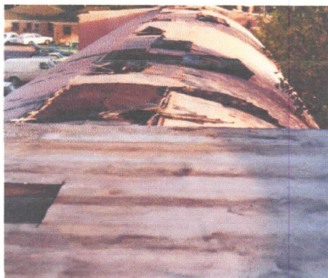
Roof damage following the fire in 1981
